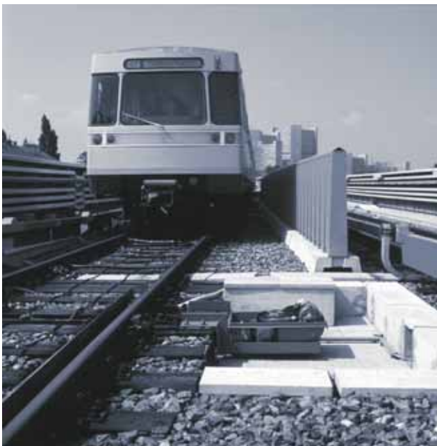
Picture 4: Points Machine along the tracks.
